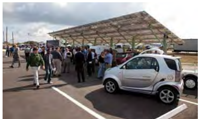
Part of the parking lot at the Propellants North facility is tailor-made for electric cars. The covered area features plug-in stations for electric vehicles. (Credit: NASA/F. Michaux)
