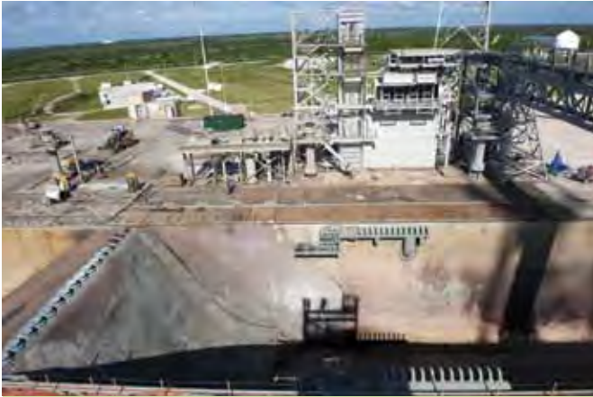
The flame trench at Launch Pad 39B, which is currently lined with fireproof bricks and concrete, will be refurbished and the flame deflector in the middle could become portable to handle future rockets of different sizes. NASA used a moveable flame trench during Apollo. (Credit: NASA/J. Grossmann)
