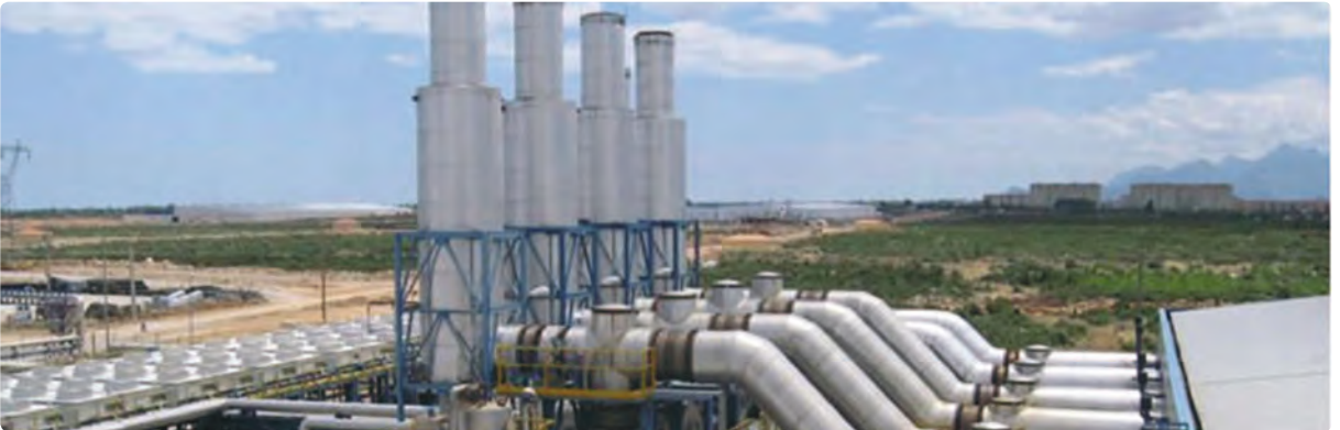
5.20: Doğal Gaz Santrali-Antalya
